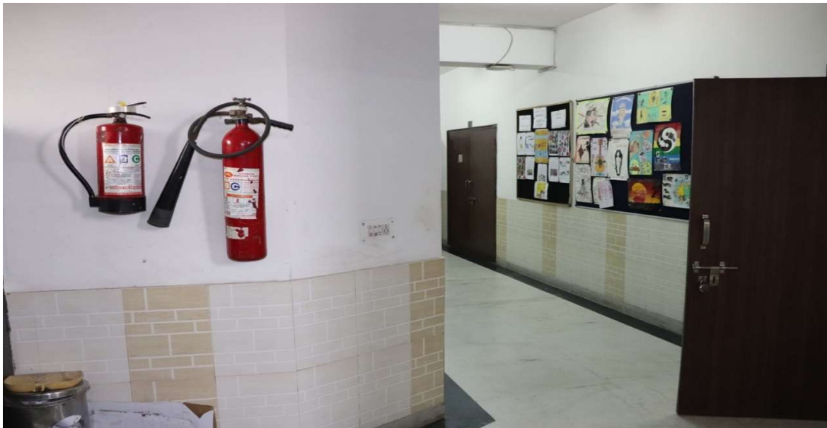
Fire extinguisher on every floor of the college
