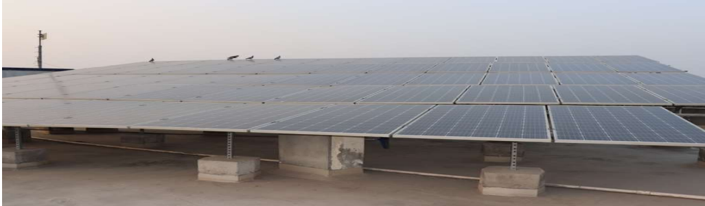
Rooftop Solar PV System
