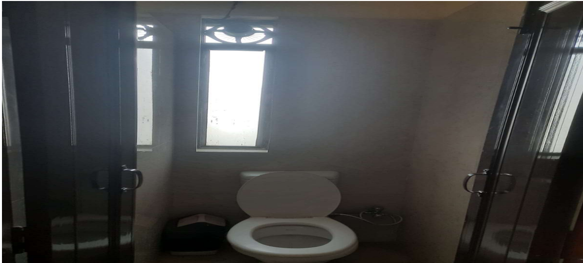
Exhaust Fan in Washrooms
