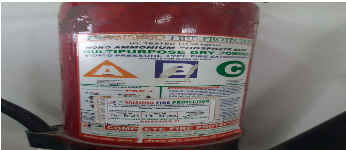
Fire extinguisher Refilling and Expiry Date
